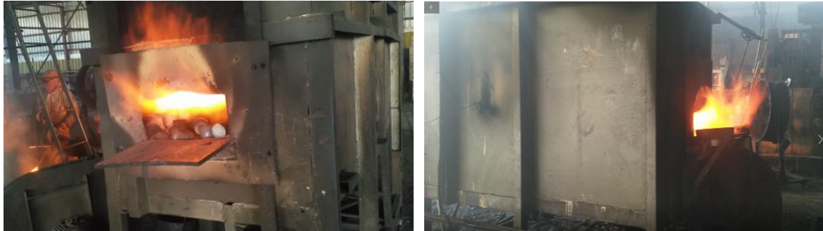
Figure 3: Oil fired furnace in operation
